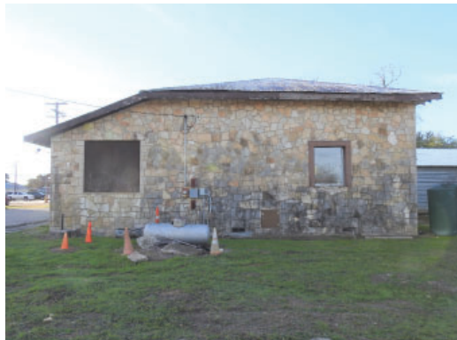
Figure 3.7: North elevation, note biological growth
