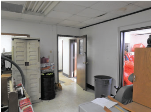
Figure 3.41: Occupied space. Note non-original VCT tile flooring, dropped ACT ceiling, and furred-out wall
