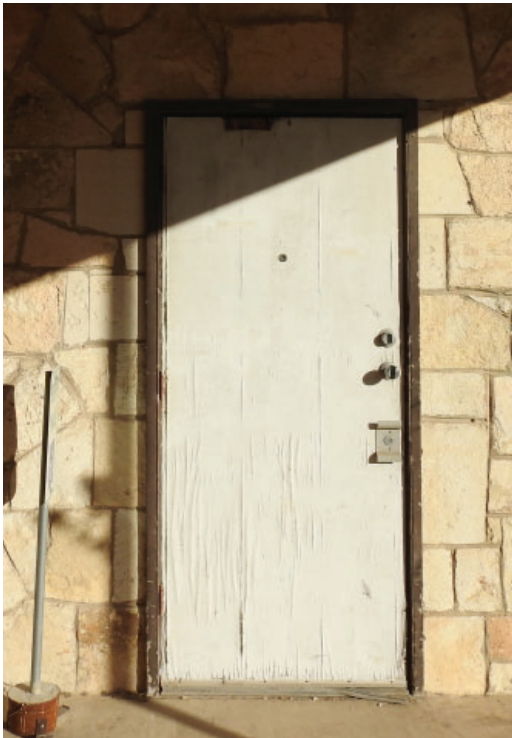
Figure 3.23: Non-original wood door in non-original masonry opening
