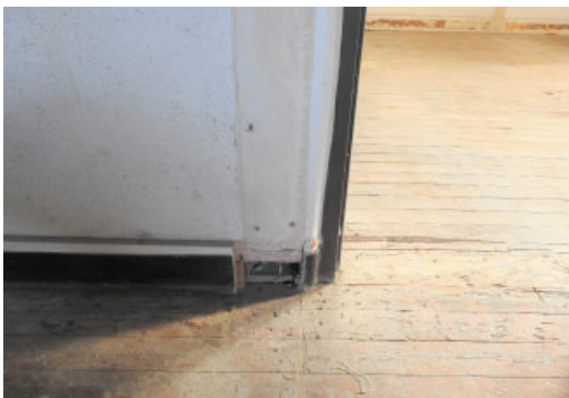
Figure 3.36: Damaged original 1"x6" wood base
