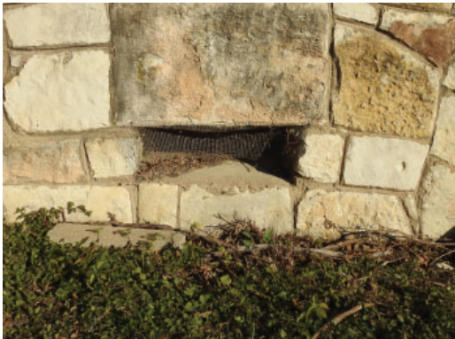
Figure 3.4: Crawl space masonry opening with damaged wire screen
