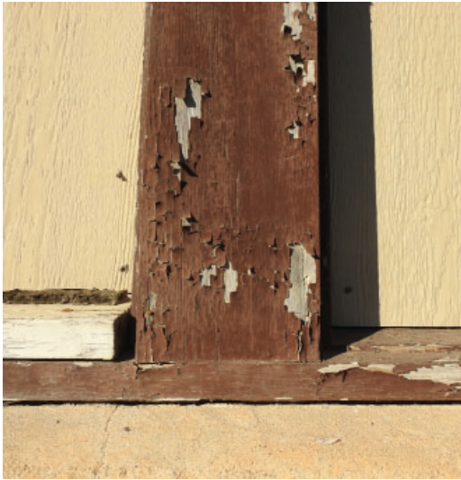
Figure 3.14: Loose paint on window frame assembly
