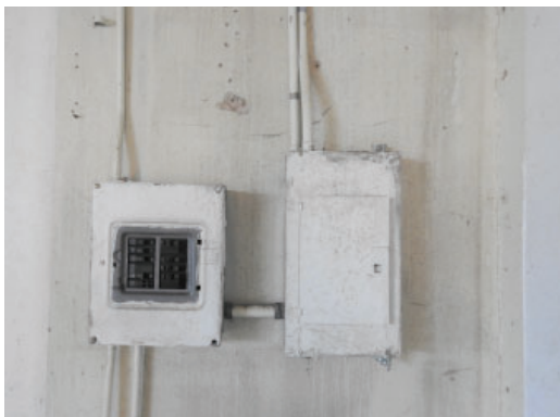
Figure 3.49: Mounted electrical equipment on back wall of stage area
