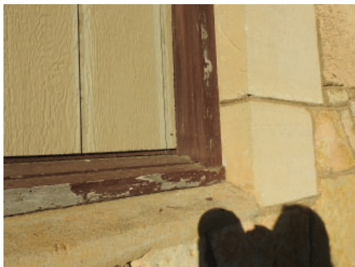
Figure 3.15: Loose paint on window frame assembly
