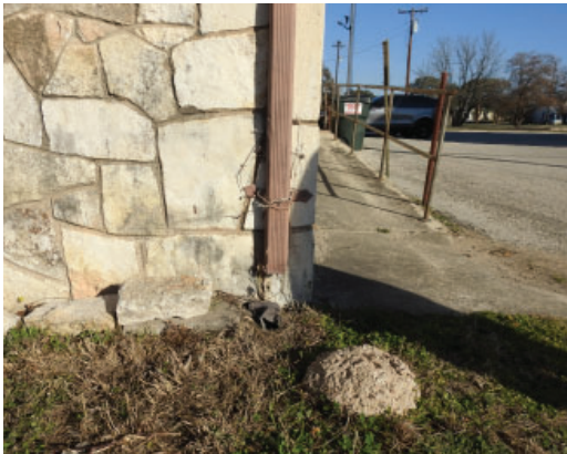
Figure 3.32: Gutter at southeast corner, note missing spout
