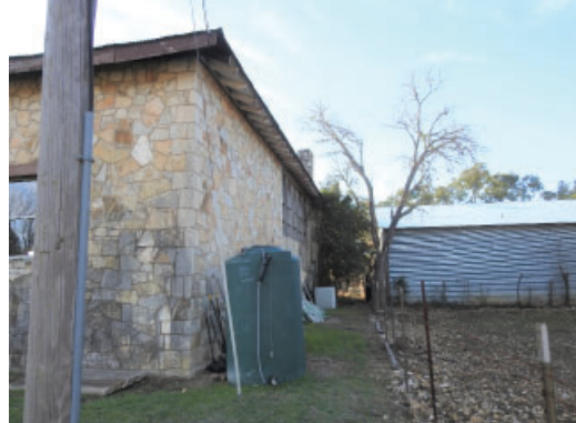
Figure 3.50: West side of building at the edge of the property. Note MEP equipment.
