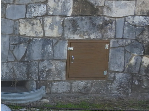
Figure 3.1: Crawl space access door, note biological growth
