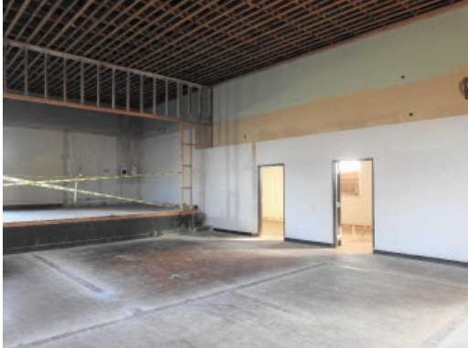
Figure 3.33: Main auditorium space. Note original wood flooring and load bearing interior wall. Stage to the left
