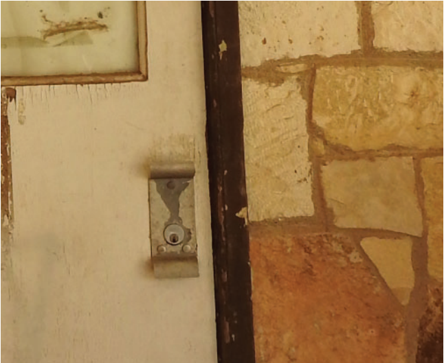
Figure 3.26: Existing hardware not compliant with ADA standards
