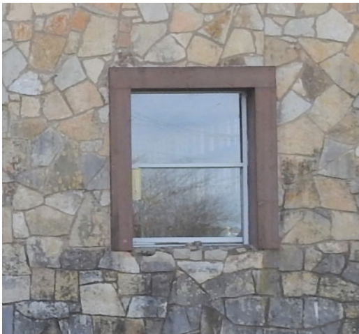
Figure 3.18: Non-original aluminum window on north elevation
